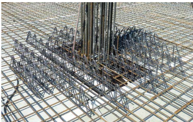
Figure 2 – This image shows the steel reinforcement for a slab around a column prior to the pouring of concrete. 1 The triangular-shaped bars improve the slab's resistance to punching shear locally around the column.
