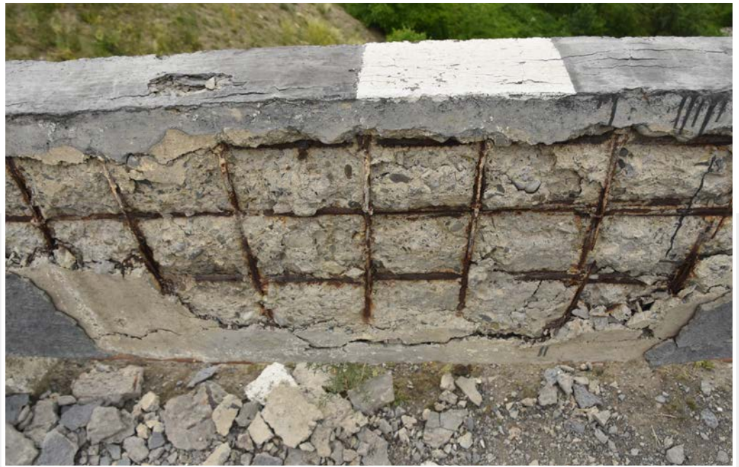
Fig.1., Chloride-induced steel reinforcement corrosion in a highway structure
